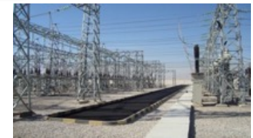
EPC-SUBSTATIONS Executed over (60) HV and MV turnkey substations up to 400 kV.
